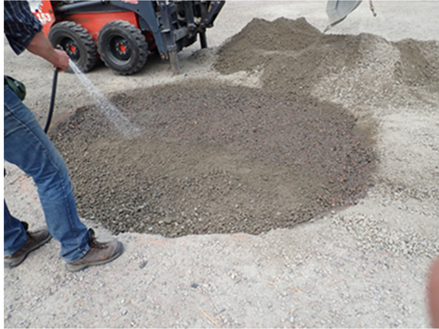
Figure 14: Watering of a fill layer using a garden hose with spray nozzles.
