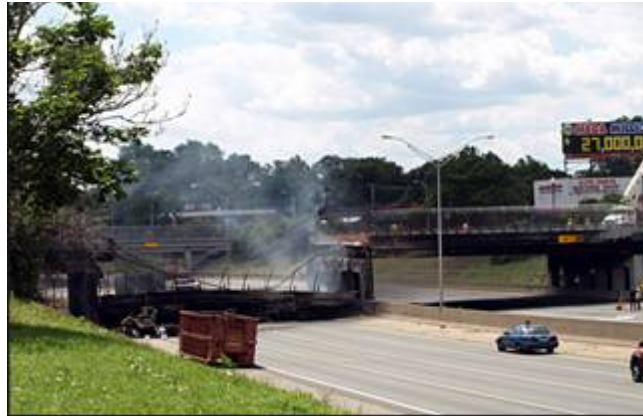
Figure 1: Collapse of the overpass bridge on I-75 due to tanker fire.
